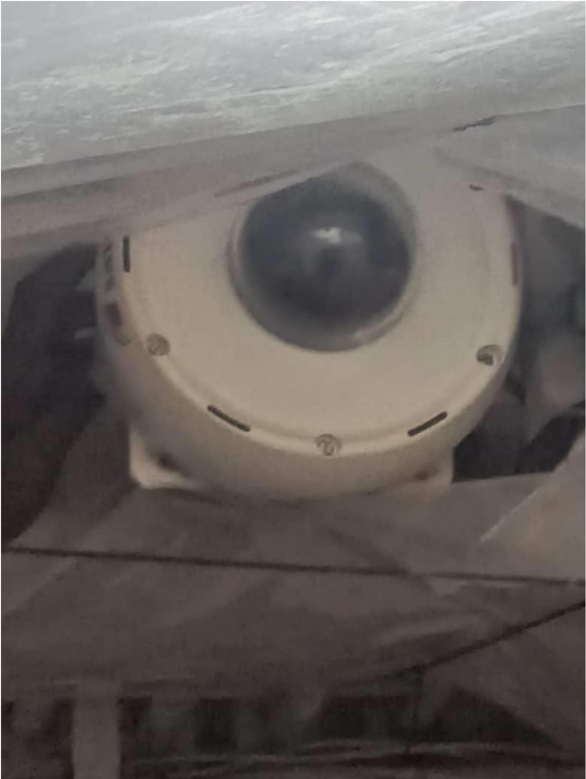
Figure 4: Close up photo of the EM camera installed in the brail room of the vessel.
