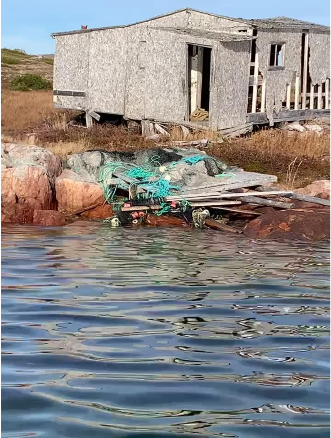
Figure 16: Collapses wharf and gear in southern 2J
