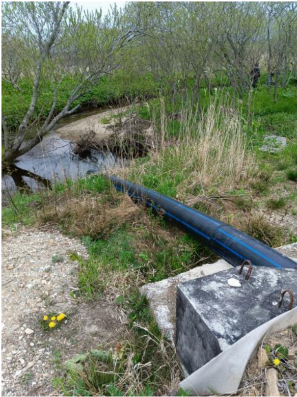
Fig. 8.1. Sewer line drain in the Luchevaya stream (basin of the Serebryanka river). May 15, 2023
