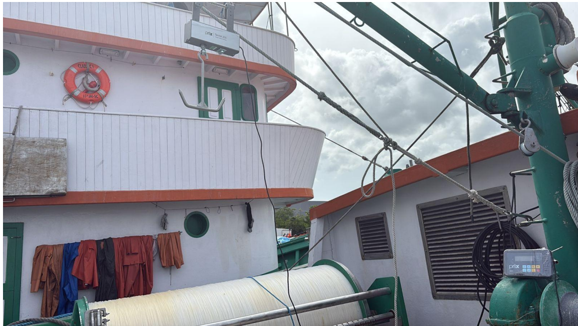
Photo of Installed Digital Scale
